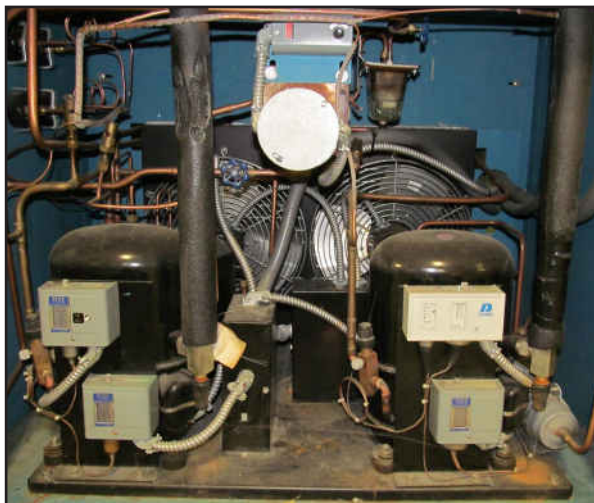
Refrigeration section of a chamber before the refurbishing process.
